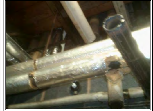
Other: Negative pipework
