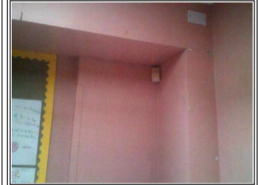
Other: Wood boxing to pipework and negative skylights
