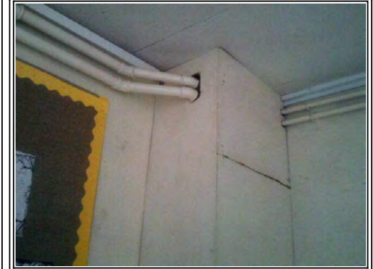
Other: Wood boxing to pipework
